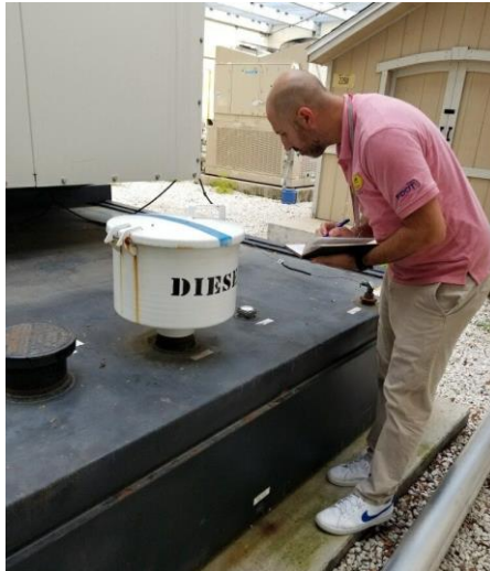
Generators and fuel ✓
